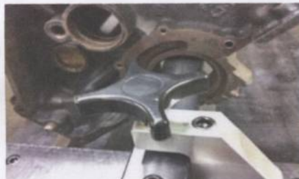
Then tighten both block bar clamps. Now you are ready to resurface.
